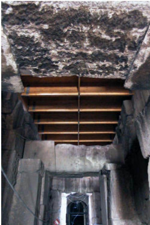
Figure 6 : Timber structures of the entrance corridor directly leaned on the travertine blocks
