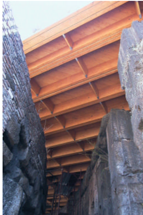
Figure 7 : Laminated wooden beams with composite reinforcements over-passing the historical masonry
