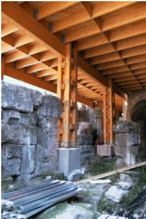
Figure 4 : Arena timber structures and the new pillars leaned on the interposed blocks
