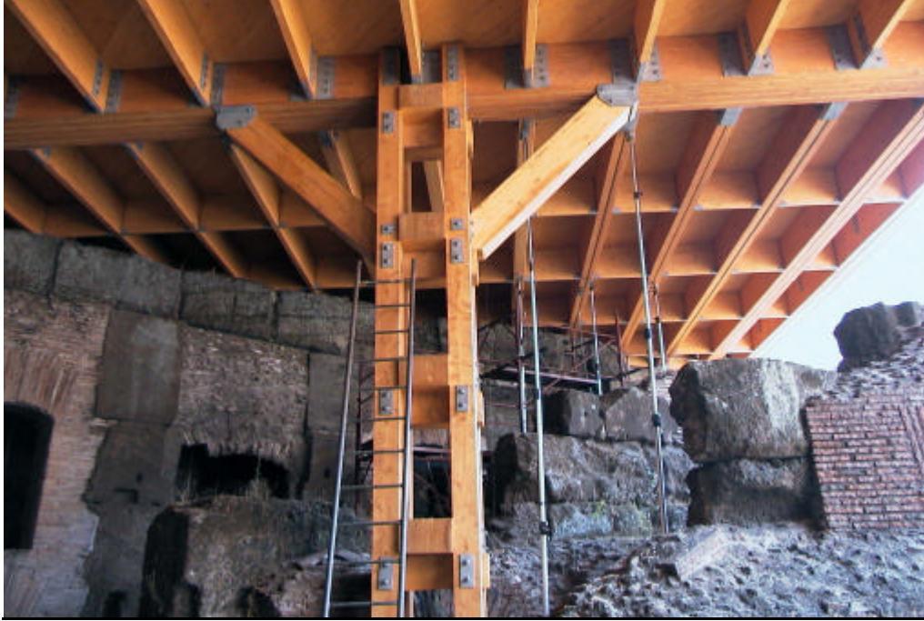
Figure 8 : The new structure in laminated wood and in composite reinforced laminated wood
